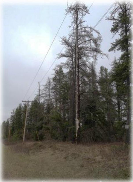
FIGURE 20 DEAD JACK PINE NEAR POWER LINE
