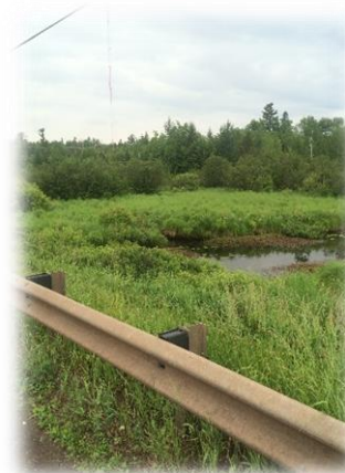
FIGURE 28 NEED FOR CULVERT, M-35/CARP RIVER CROSSING
